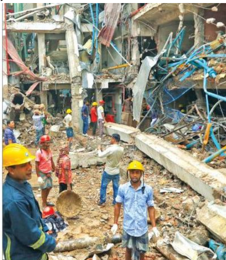
The remains of the building of Multi Fabs Limited after a boiler explosion. Photo: Prothom Alo, 7 July 2017.
